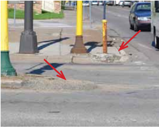
Curb ramp is blocked by post, and median intrudes into the crosswalk along the southern edge of Broadway Avenue, near Sheridan Elementary School.
