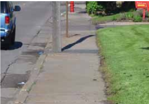
Narrow sidewalks with obstructions make walking along Broadway Street NE less pleasant and inviting than it could be.
