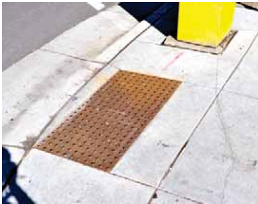
Pedestrian ramps should have detectable warning curb features for additional safety and ADA compliance.
